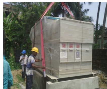
Figure 13 Compact Secondary Substations (CSS)
