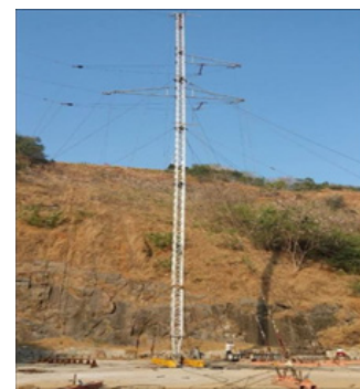
Figure 9 220kV ERS Towers
