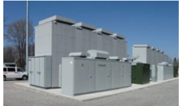
Figure 19 battery-based energy storage system
