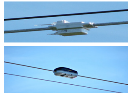
Figure 27 DLR in Power Line
