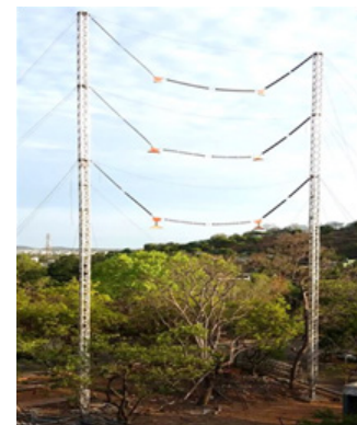
Figure 10 400kV ERS Towers
