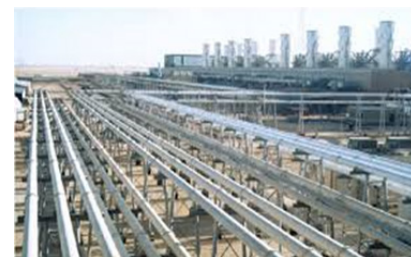
Figure 28 Gas Insulated Lines
