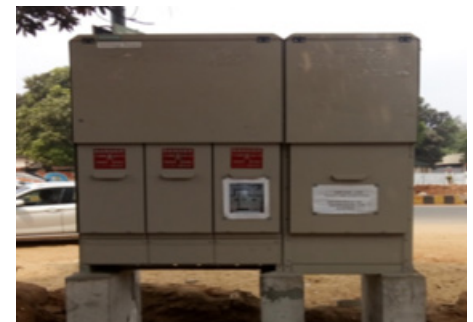
Figure 12 Ring Main Units
