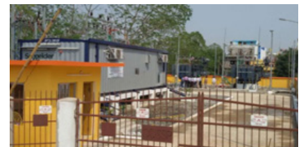
Figure 18 E-house at Unit-2, Bhubaneswar under TPCODL
