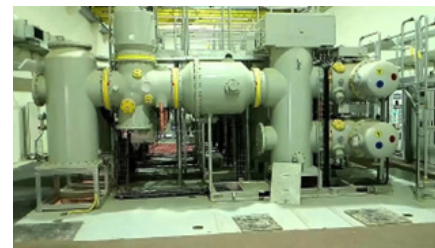
Figure 16 220/132kV Gas Insulated Substations
