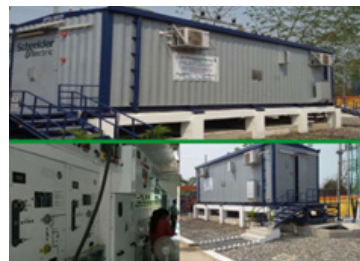
Figure 17 E-house at Bhubaneswar
